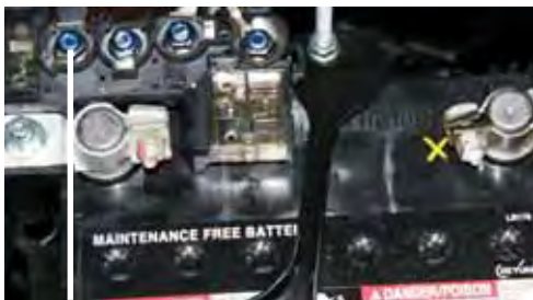
DC to DC Converter Cable Connection
